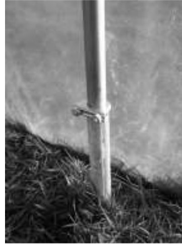
Clamping the hoop into position at the top of the foundation tube.
