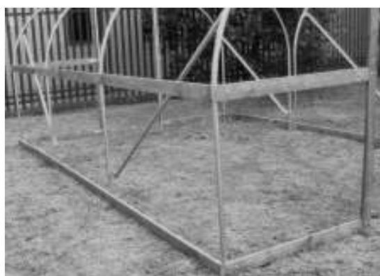
Fig60 – Base Rail at ground level. Side Rail at top of straight side.
