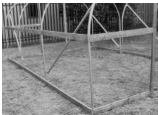
Fig41 – Base Rail at ground level. Side Rail at top of straight side.
