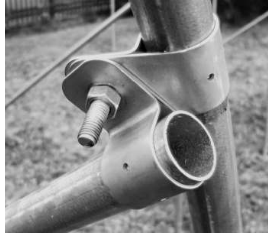
*Wrong clamp position - Protuding outside the end hoop.
